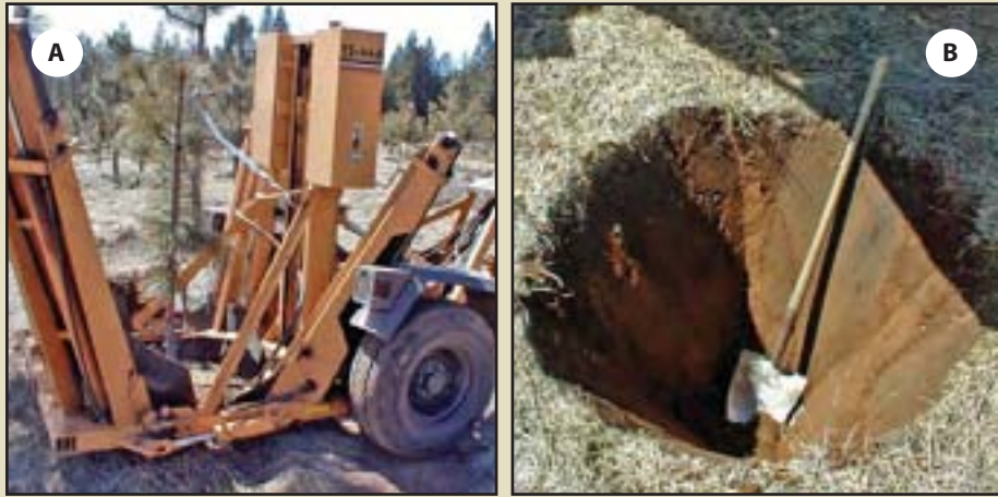
Figure 10.61 – Mechanical tree spades (A) can extract large plants quickly. A planting hole must be excavated prior to transplanting (B) and this can be accomplished with a tree spade. Photo credit: Chris Jensen, USFS.
