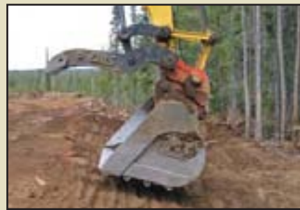
Figure 10.12 – An alternative form of imprinting road cuts and fills that does not compact soils is welding angle iron onto the bucket of an excavator. As the excavator pulls topsoil into place and contours the slope, it presses the face of the bucket into the soil surface to form surface imprints.
