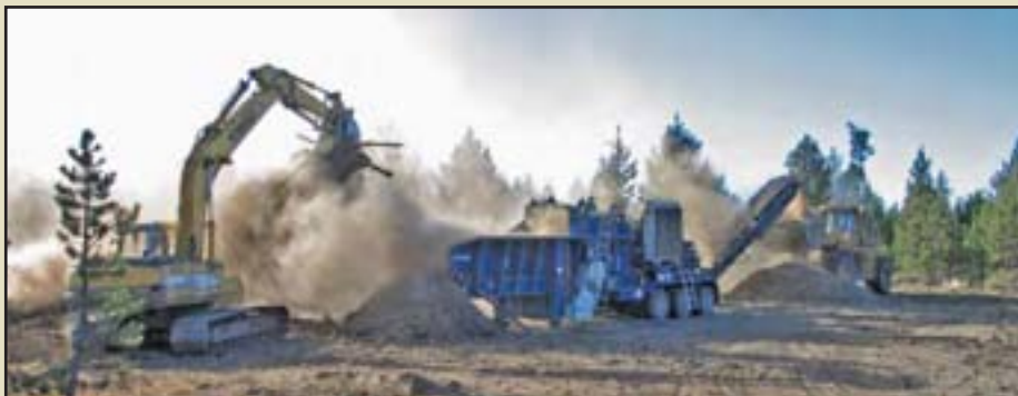
Figure 10.19 – Large mulching operations require access and working space. The operation shown in this photograph shows the wood waste material being dropped into a grinder with an excavator (left), and conveyed as mulch to the bucket of a front end loader (right).
