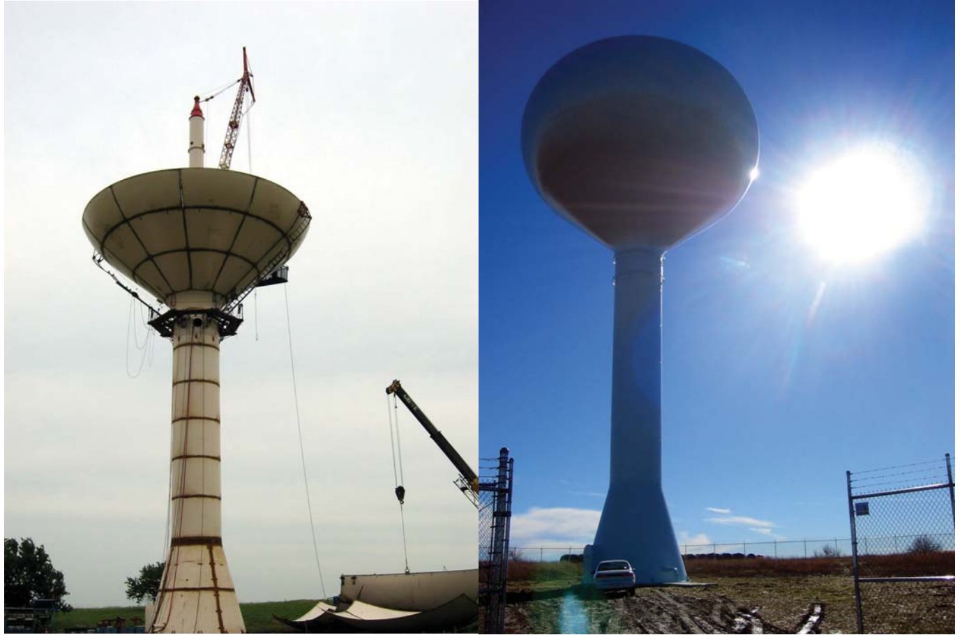
These photographs show the construction and completion of a tank in Bartlesville, Oklahoma.
