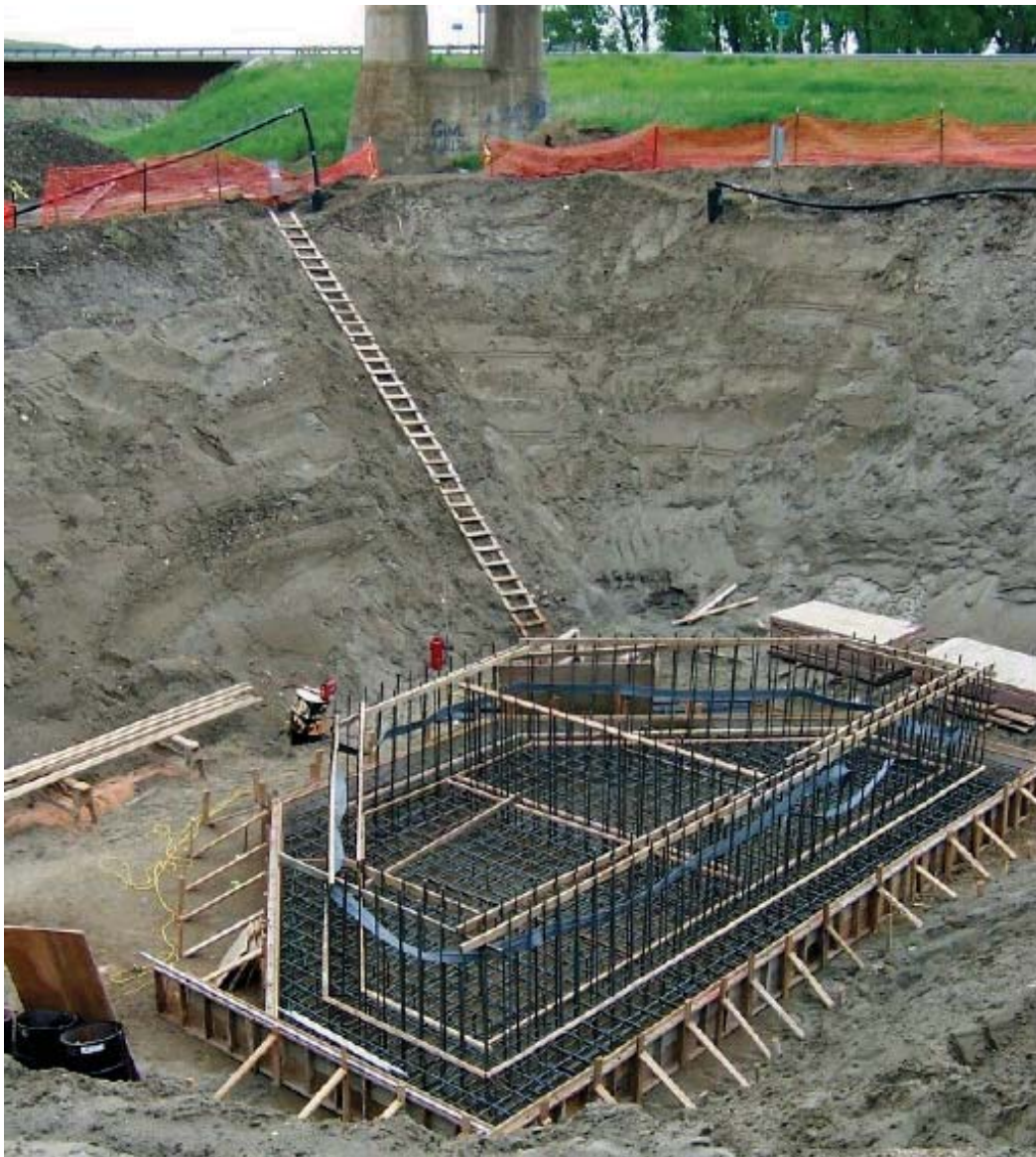
Fort Peck-Dry Prairie Regional Water System. This raw water intake pump station will draw an average daily flow of 5.5 million gallons per day (MGD) from the Missouri River to serve 22 communities in northeastern Montana. These communities are currently served by individual wells with poor water quality.
