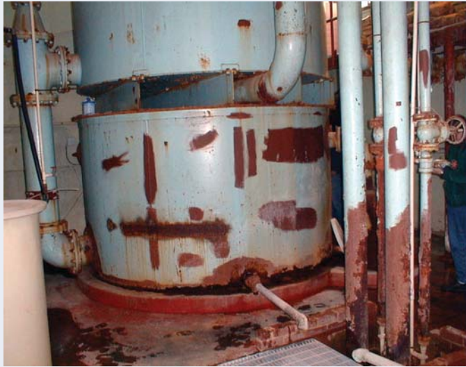
This corroded, valveless filter is badly in need of replacement.
