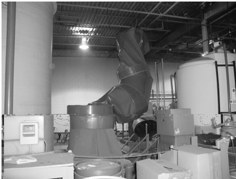
Figure 8. Collapsed 36-inch-diameter main header at scrubber along east wall.
