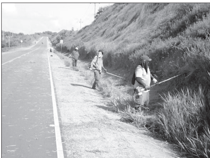
Figure 12: Grass-Cutting Crews and Damaged Guardrail
