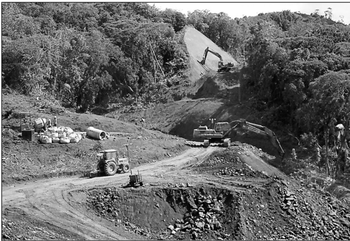
Figure 10: Compact Road Construction Terrain and Cut Slope Failure
