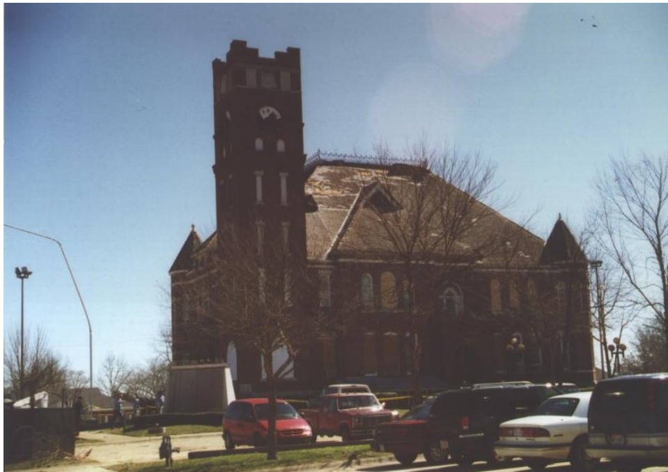
IB: DOD 6: Uplift of light-weight roof deck and insulation; significant loss of roofing material (>20%)
