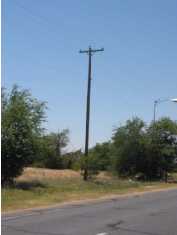
ETL: Single Wood Pole
