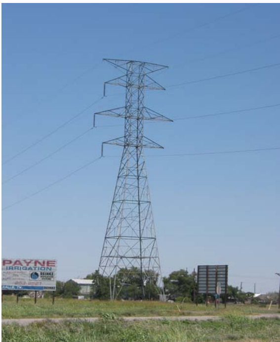
ETL: Metal Truss Tower
