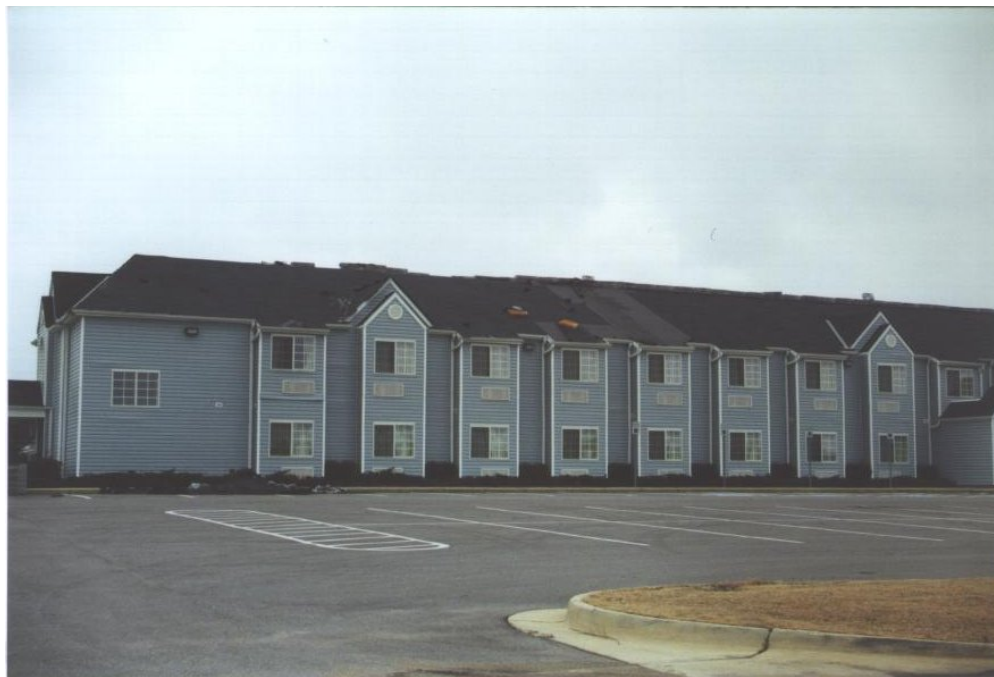
ACT: DOD 2: Loss of roof covering (<20%)
