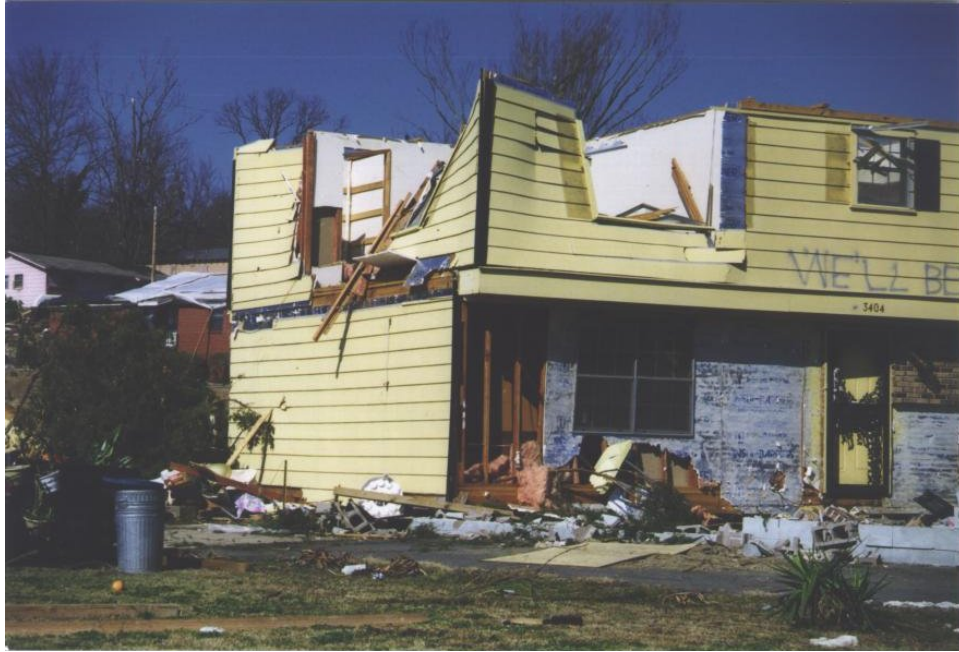
ACT: DOD 4: Uplift or collapse of roof structure leaving most walls standing
