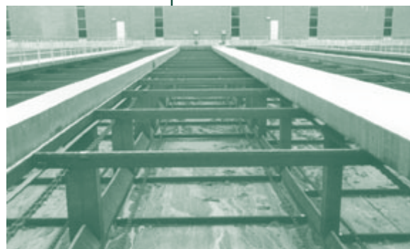
Southeast Water Pollution Control Plant
