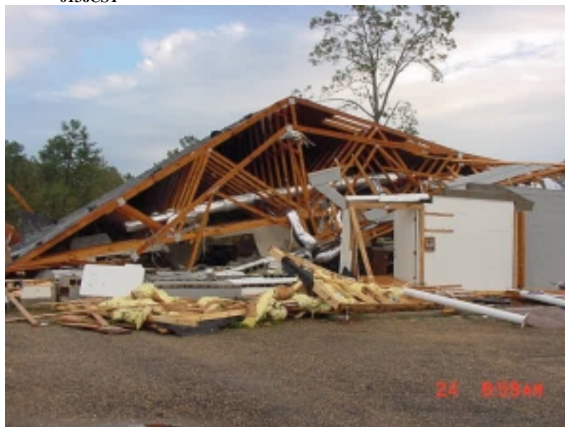
Damage to the VFW building north of Magee.
