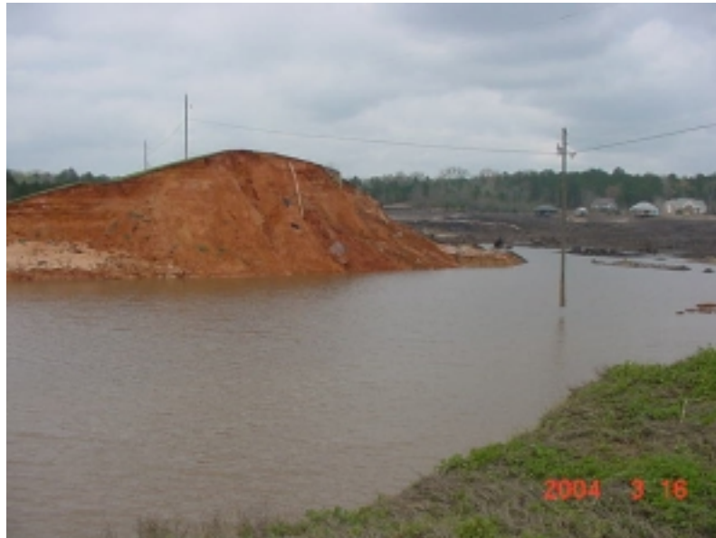
The breach in the Big Bay Lake dam.
