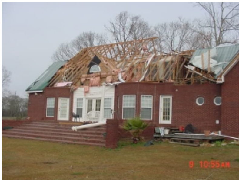
Roof blown off house north of Purvis.
