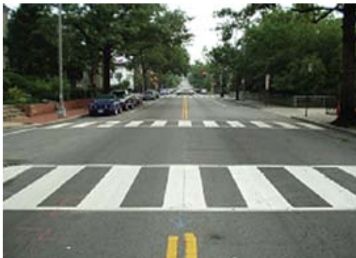
High-visibility crosswalks have thick markings that are easy for approaching drivers to see. Pictured is a ladder type crosswalk marking.
