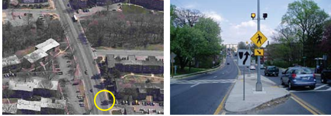
These pictures show a location where a median crossing island was installed to improve the safety of pedestrians accessing a well-used bus stop on a busy, high-speed roadway. The photo on the left was taken before and the photo on the right was taken after the improvement was made.
