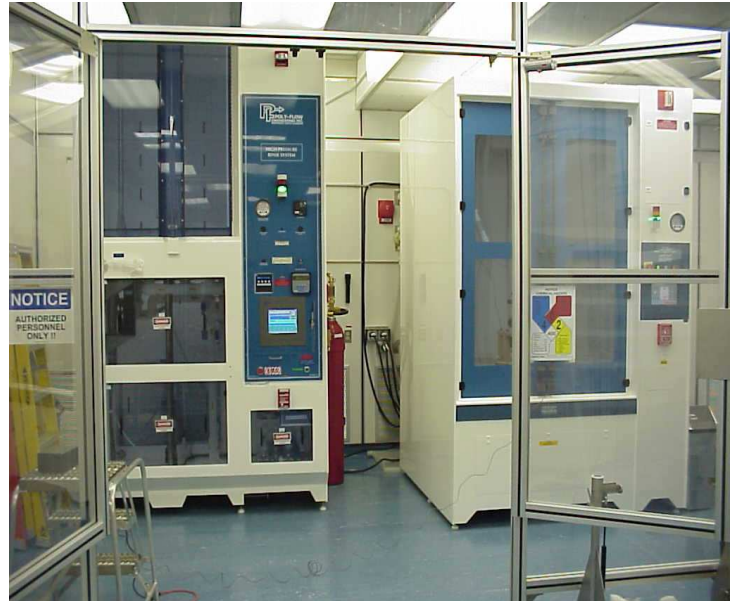
Closed chemistry and high-pressure rinse cabinets in the clean room
