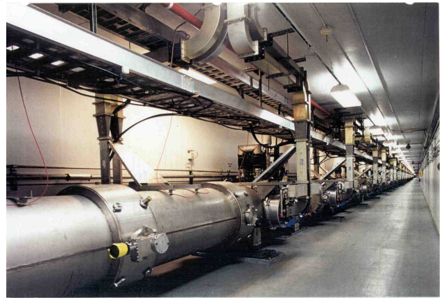
Cryomodules in the accelerator tunnel
