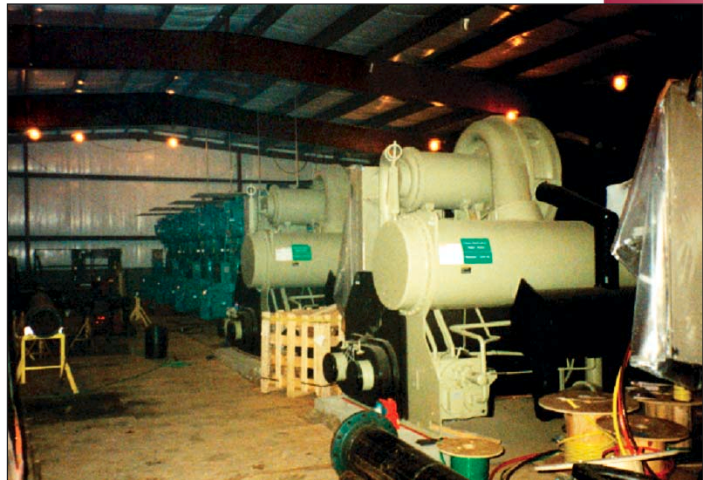
Fort Knox's Army Ireland Hospital represented a major conservation project involving a $4.8 million boiler-chiller replacement.
