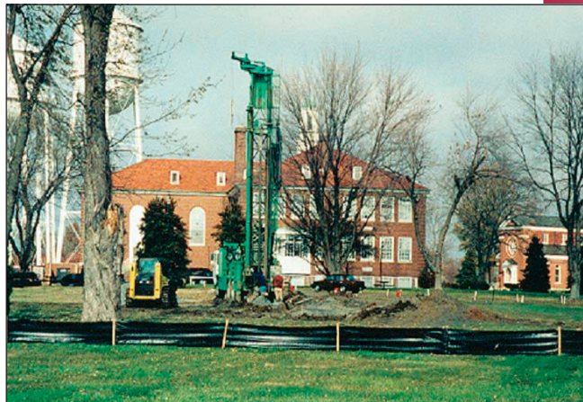
Geothermal heating and cooling was installed in some buildings to save energy at the base.
