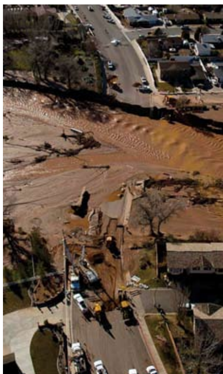
Figure 1. Bridge washed out by the Santa Clara River in St. George, Utah, January 2005. (Photo by Trent Nelson, Salt Lake Tribune).
