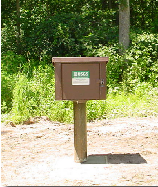
Figure 4. A newly installed USGS monitoring well used for measuring ground-water levels and water-quality in Michigan. (Photograph by Charles Whited; U.S. Geological Survey.)
