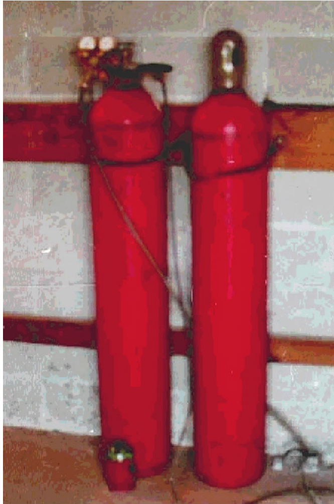
Figure K-2 - Properly Secured Cylinders
