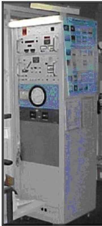
Figure B-6 - Master Control Console (Full Rack Assembly)
