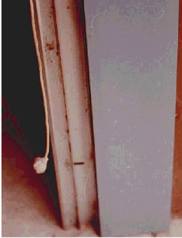
Figure K-3 - Ungrounded Overhead Door Railing
