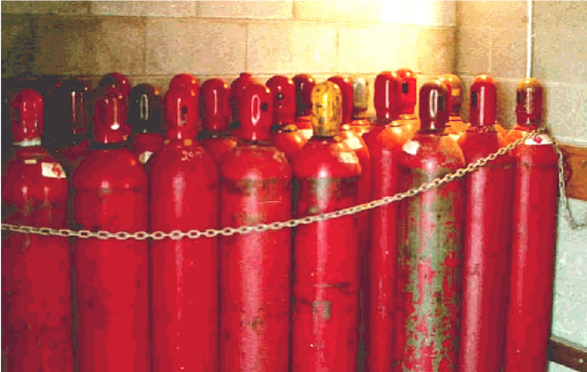
Figure K-1 - Cylinders Secured Improperly
