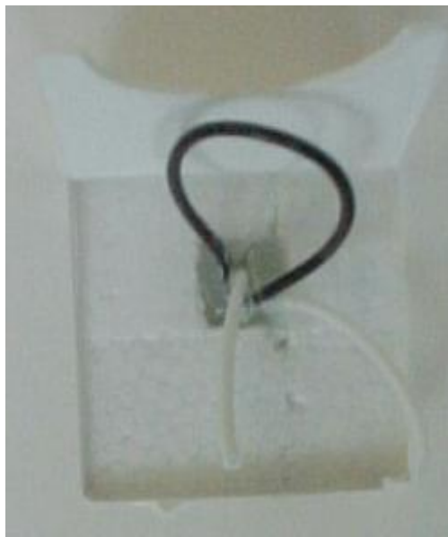
Figure N-9 – Cut Wires
