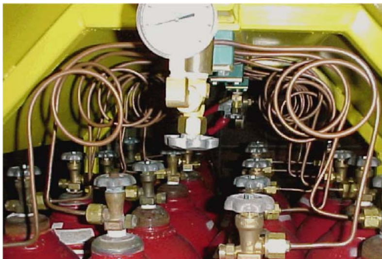
Figure K-6 - Unauthorized Manifolding of Cylinders
