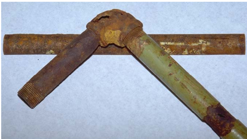
FIGURE III-23 POOR CONSTRUCTION PRACTICE
