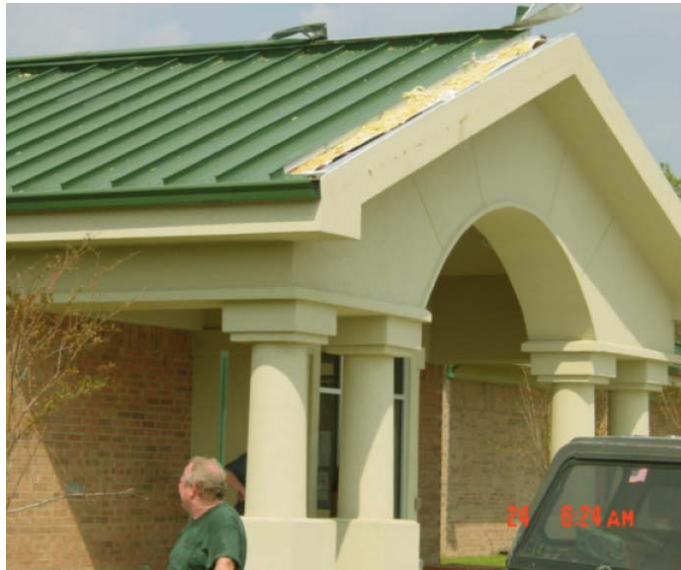
Figure 5: Damage to the roof, Gulfport, Mississippi, District Office
