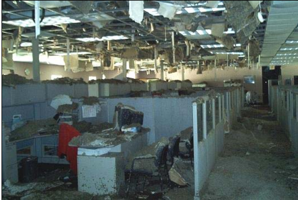
Figure 6: Inside the Kenner, Louisiana, District Office
