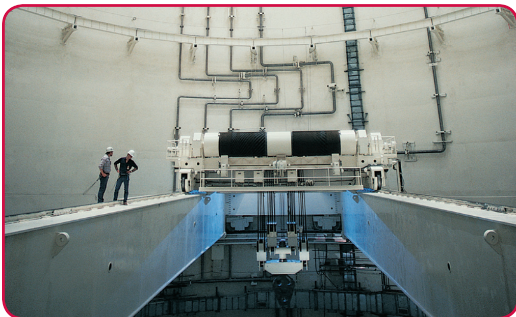
Inside a nuclear reactor containment building
