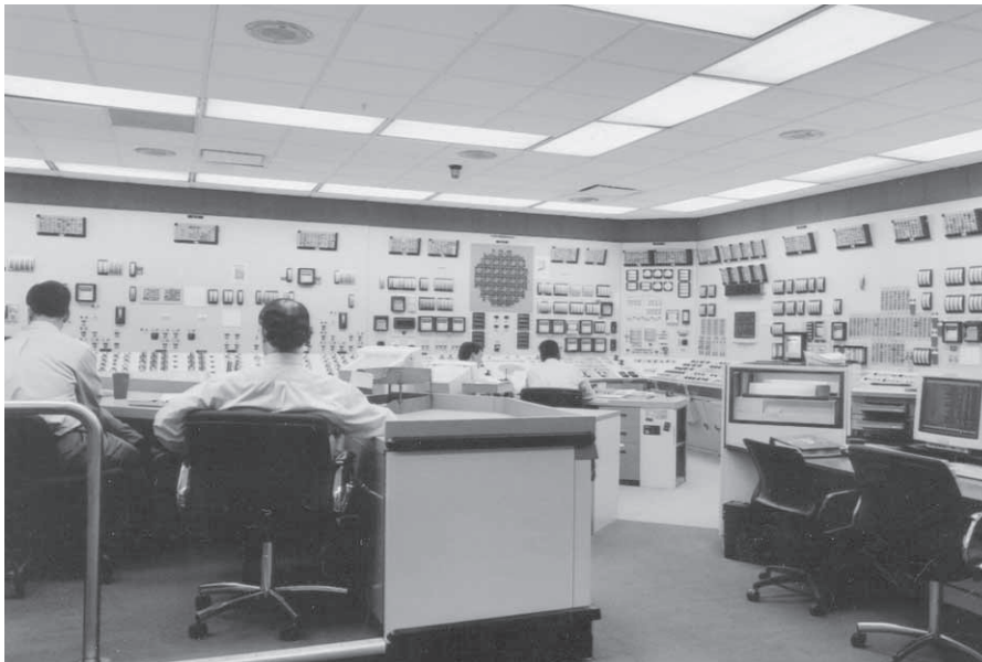
Control Room at a Nuclear Power Plant
