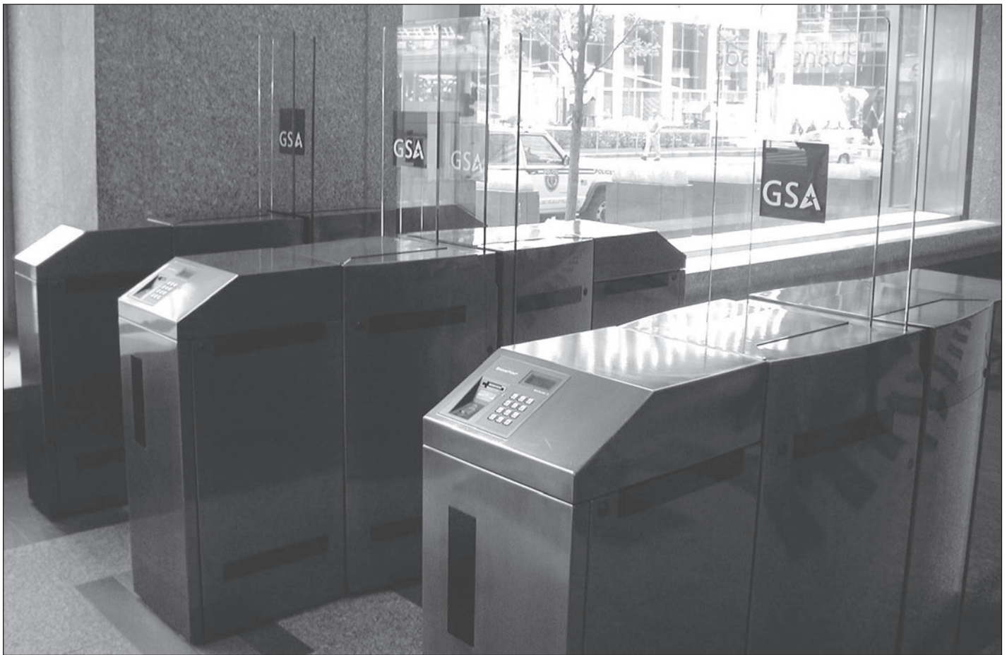
Figure 1: Smart Card Access Portals at a Federal Building Entrance
