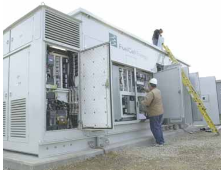
Technicians complete work on a fuel cell that will supply electricity to nearby homes. The Westerville, Ohio Fuel Cell Demonstration Project is the only known application of a fuel cell in which the electricity produced is patched in to the power grid for general consumption.
