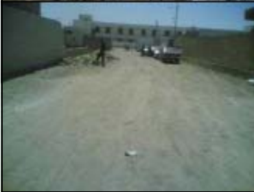
A road repair project funded by an ITI grant restored the community's streets, eliminated unsanitary conditions, and provided over 3,000 temporary jobs.
