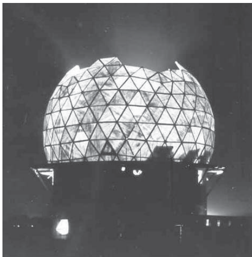
FIG. 9. Nighttime view of the radome on NSSL's Cimarron Doppler radar building being assembled by the Oklahoma Air National Guard in 1973. [NSSL photo by Charles Clark.]
