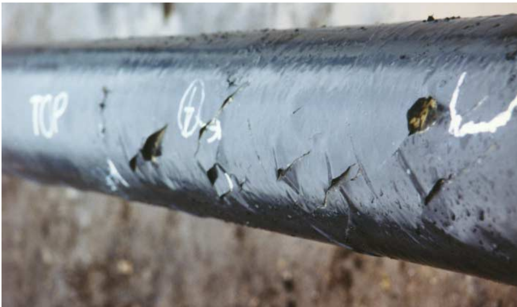
Figure 8. Cracks in the tape coating on 8-inch pipe excavated at accident site
