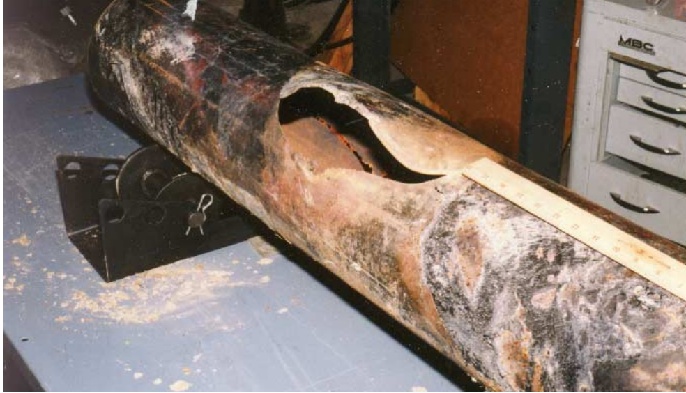
Figure 5. Pipe section containing 12.5-inch rupture
