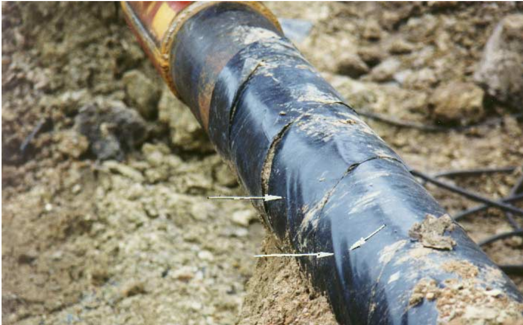
Figure 7. Disbonded tape coating on 8-inch pipe extracted at accident site (Arrows show disbonded area under tape coating.)
