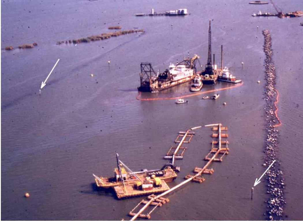
Figure 3. Aerial view of the stern of dredge Dave Blackburn (large white vessel near the center) and the pilings (marked by arrows) that were believed to locate the pipeline. The rectangular framework on the stern of the dredge is directly over the ruptured pipeline.
