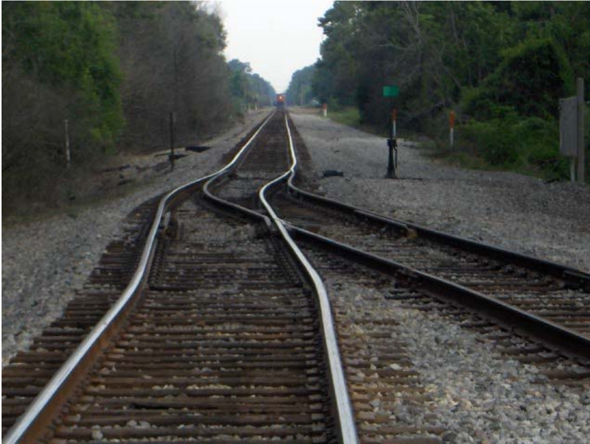
Figure 1. Looking south along the section of misaligned track encountered by the Amtrak train.
