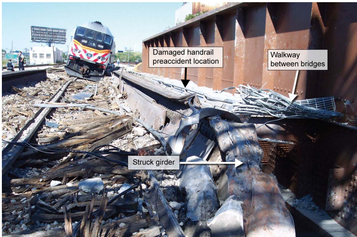
Figure 4. Damage to the 47th Street Bridge and adjacent walkway and handrail.
