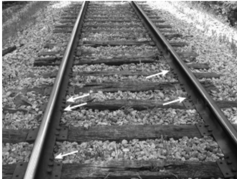
Figure 7. Ties with few anchors, indicated by arrows.
