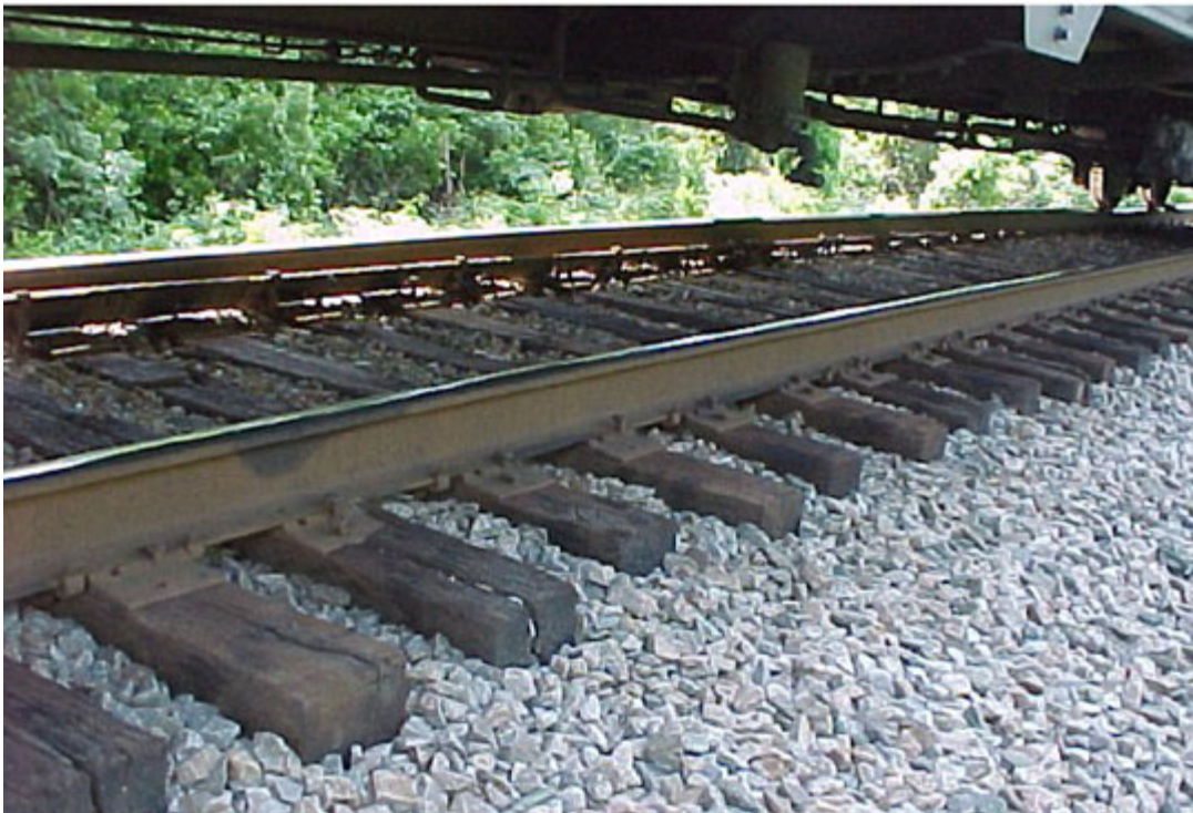
Figure 8. Ballast conditions in accident curve.
