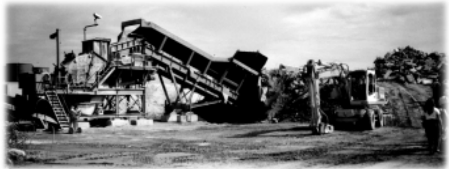
Pictured here is a concrete crusher at the Jean Lefebvre Inc. reclaiming facility in Pontblon, France. Concrete from pavement and building slabs and construction and demolition wastes are processed and sorted into many aggregate gradations. The final product is widely used in road construction in France.
