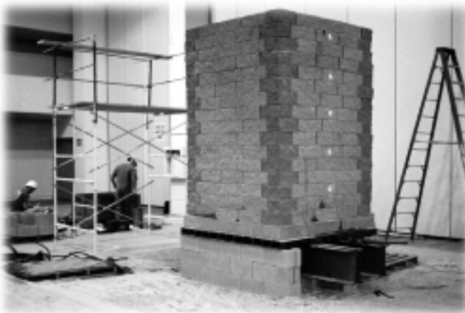
This GRS mass was constructed and load tested at the Masonry EXPO 2000 in Las Vegas, NV.
