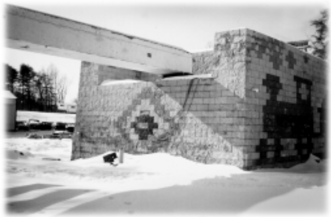
This recently completed full-scale GRS embankment/abutment project, located at TFHRC, was completed in April 1999.
