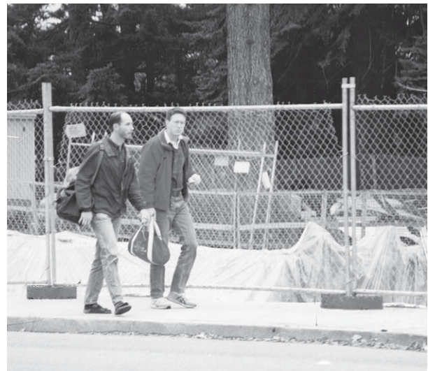
Fencing used to secure a work area supported by blocks needs to be positioned to avoid creating obstacles or tripping hazards for pedestrians.
