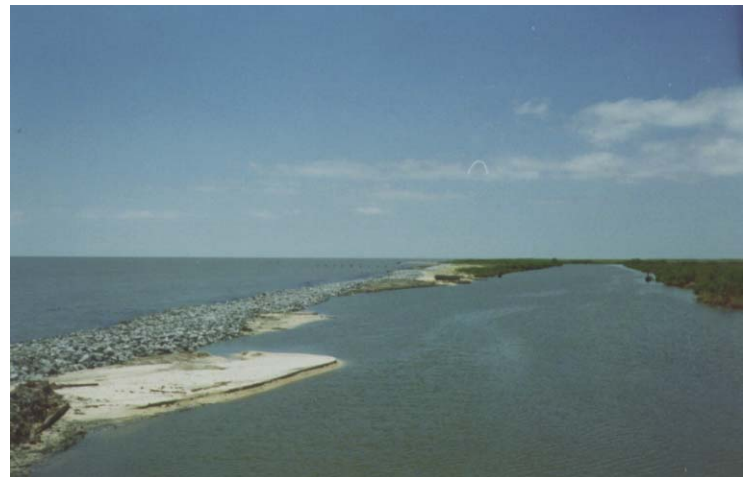
This section of Mobil Canal was backfilled and armored with rock to reestablish the separation between the canal and the gulf so that salt water would be prevented from damaging the intermediate marshes in the interior of the island.
