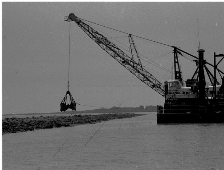
The proposed terraces at Four Mile Canal will be constructed in a similar fashion as shown above. The above photo is of the Captain Buford Berry constructing terraces at the project at Little Vermilion Bay (TV-12).
