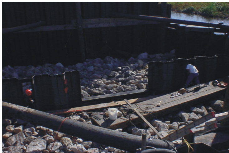
This picture was taken during installation of the self-regulating tidegate (SRT). Fish slots on either side of the SRT will allow movement of marine life between the areas when the gate is closed.
