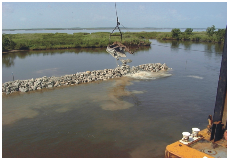
Above is the rock dike under construction. A large open water area is in the background.
