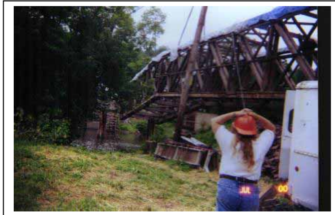
Figure 178. How NOT to relocate a covered bridge for repair work.
