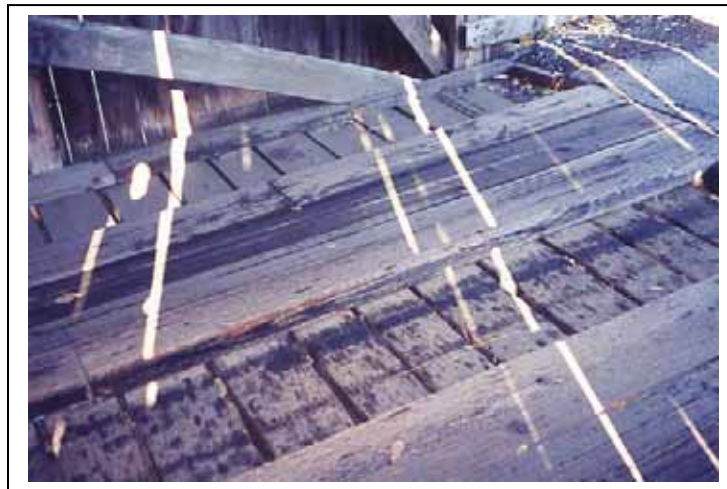
Figure 46. Typical transverse plank decking with running planks—Salisbury Center Bridge, Herkimer County, NY.
