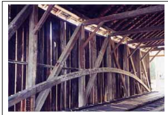
Figure 93. A lightweight arch attached only to the inside of the truss–Salisbury Center Bridge, Herkimer County, NY.
