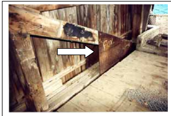
Figure 156. Steel plates at heel connection of queenpost truss—Power House Bridge, Johnson, VT, before its collapse in 2001.
