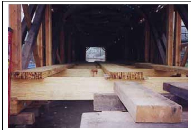
Figure 48. Glue-laminated floor beams and decking system under construction—Hamden Bridge, Delaware County, NY.
