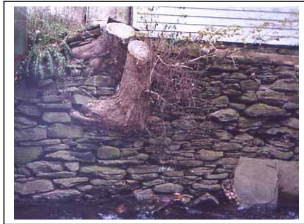
Figure 72. Damage to stone wall caused by tree roots.
