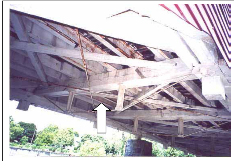
Figure 159. Installation of metalwork beneath a timber floor beam—Wehr Bridge, Lehigh County, PA.
