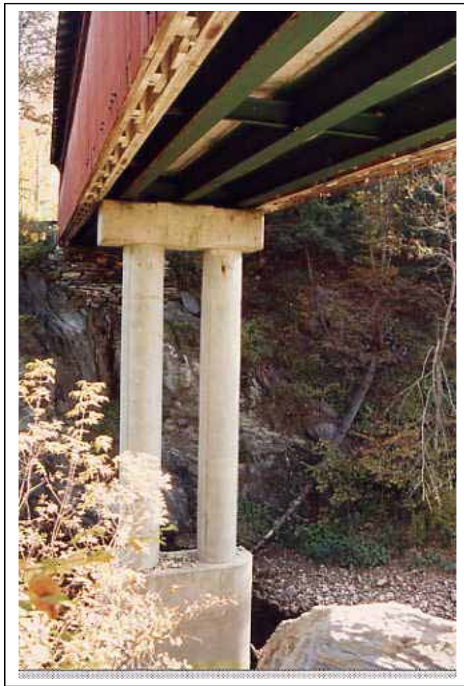
Figure 50. Independent floor system—Chiselville Bridge, VT. Note that the pier cap does not support the timber truss, which must still support the weight of the covering and snow.
