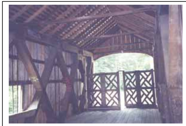
Figure 97. No X lateral system and no knee braces—Comstock Bridge, East Hampton, CT.
