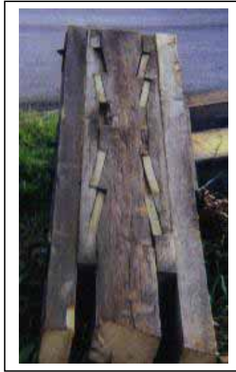
Figure 180. A classic “Bolt-of-Lightning” splice. It relies on end bearing and shear to transfer the forces. The cuts include vertical mitering to allow the bearing blocks to settle into a tight fit, without falling out, should the joint tend to stretch
