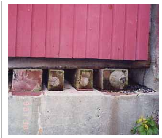
Figure 166. Sacrificial timbers beneath truss elements.
