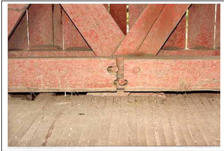
Figure 143. A chord butt joint in trouble—Station Bridge in Northfield, VT.
