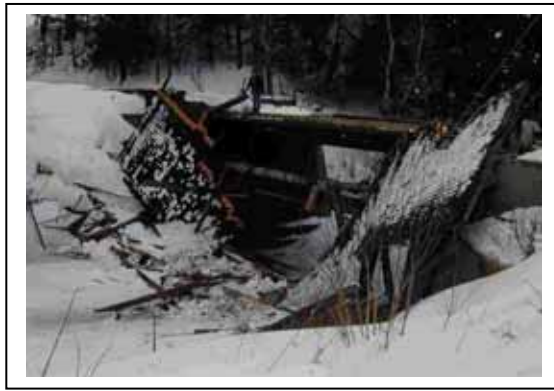
Figure 254. Bridge after collapse from snow.
