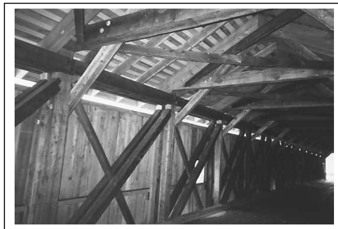
Figure 98. An extremely strong upper lateral and knee brace system—Hamden Bridge, Delaware County, NY.
