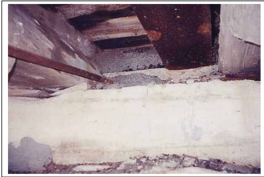
Figure 167. Accumulation of debris and asphalt encasing timber elements.
