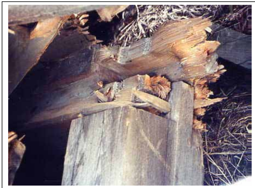
Figure 137. Tie beam to top chord connection details of failed joint.
