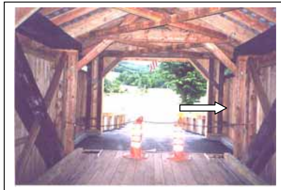
Figure 15. A shelter panel separate from the trusses—Hamden Bridge, Delaware County, NY.
