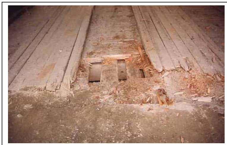
Figure 164. Consequences of the poor entrance drainage in figure 163.
