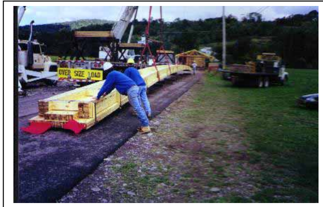
Figure 181. One-hundred-thirty-foot- (39.6 meter) long one-piece bottom chords—monsters to fabricate and deliver and a handful to work with.
