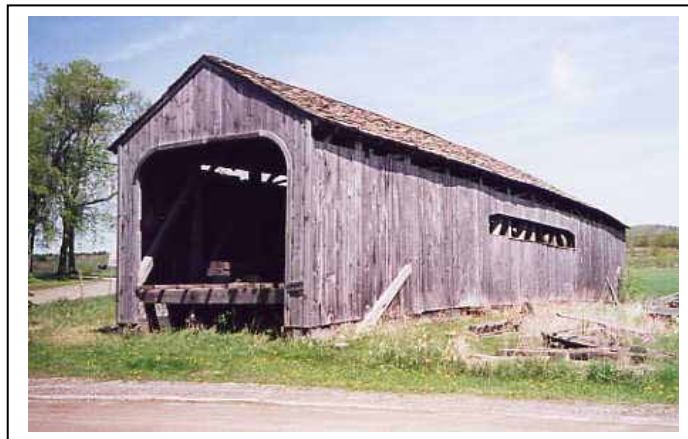
Figure 81. Example of bridge without protective treatment (the Westford Bridge in Vermont before its recent rehabilitation).
