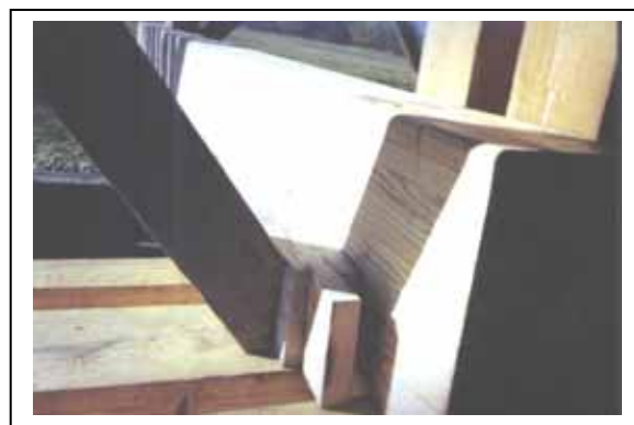
Figure 185. Typical “folding wedges” of a counter. In this application, the main (glue-laminated) transverse member in the middle of the photo is the Floor Beam. The counter on the left bears against the wedges, then the Floor Beam against the side of the post.
