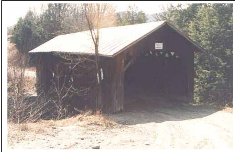
Figure 163. Unfortunate approach grading directing drainage into a covered bridge—West Hill Bridge, Montgomery, VT.
