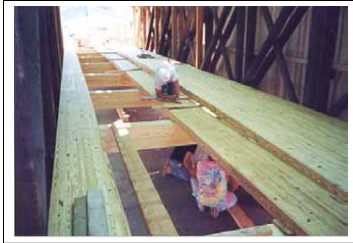
Figure 160. Strengthening by using glue-laminated deck panels and floor beams—Hamden Bridge, Delaware County, NY.
