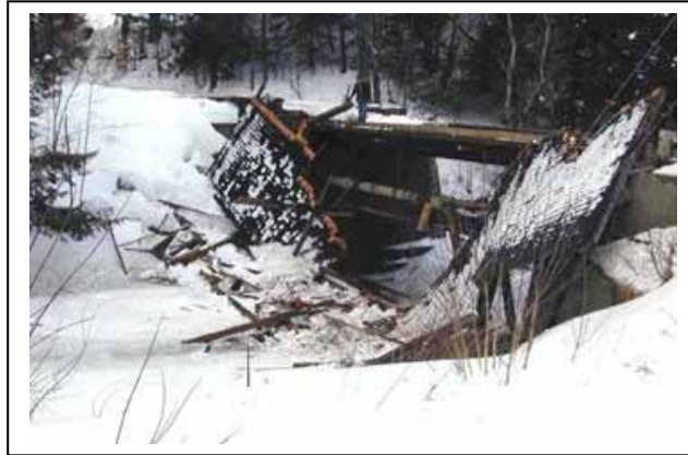
Figure 85. Snow load on covered bridges can cause failure—Power House Bridge, Johnson, VT.
