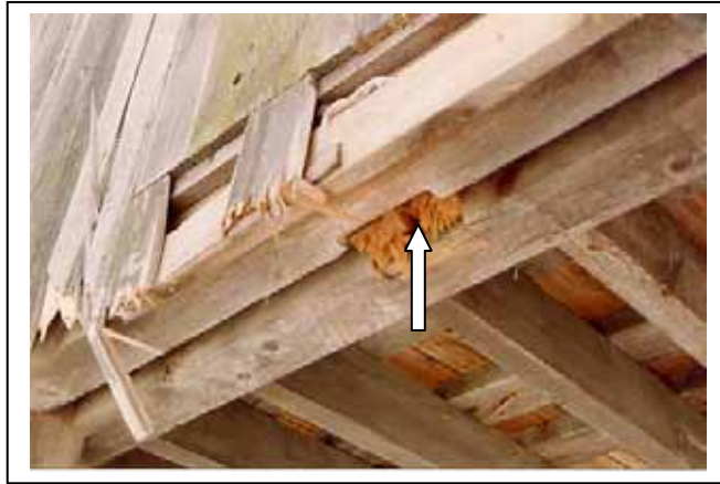
Figure 30. Example of a broken tail from ice impact—South Randolph Bridge, VT.
