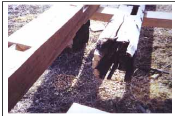
Figure 205. Hidden rot inside top of old post.
