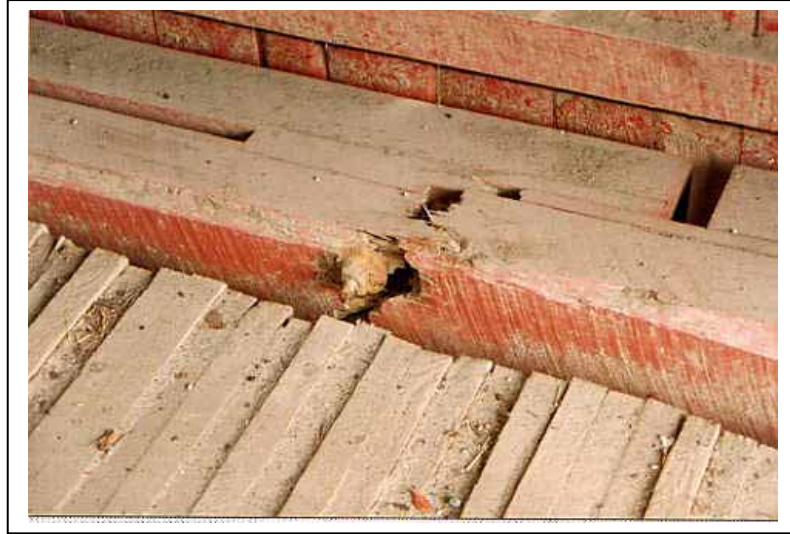
Figure 101. Example of a tensile failure of a bottom chord in a covered bridge.
