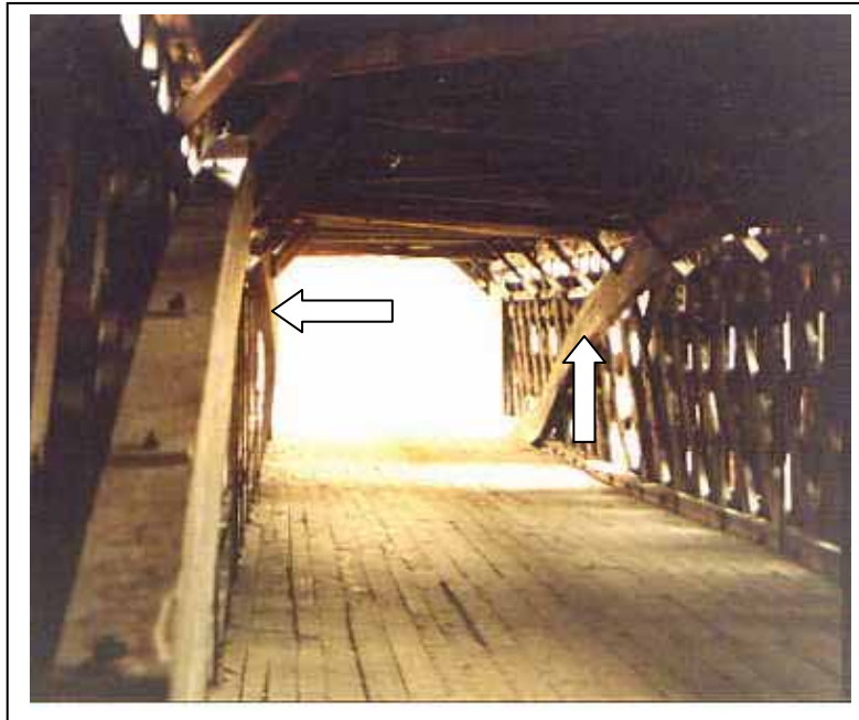
Figure 154. An arch element added to a Town lattice structure—Scott Bridge, Townshend, VT.
