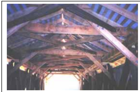
Figure 182. Internal bracing. It is certainly hard to pick out, but the major light-colored diagonal member is the Knee Brace. It is bolted to a lighter color Tie Beam and behind it with a Principal Rafter. The darker members are the original upper lateral system.
