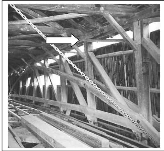
Figure 89. Typical eccentric joint in a timber truss (Brown's River Bridge, Westford, VT, before its recent rehabilitation).
