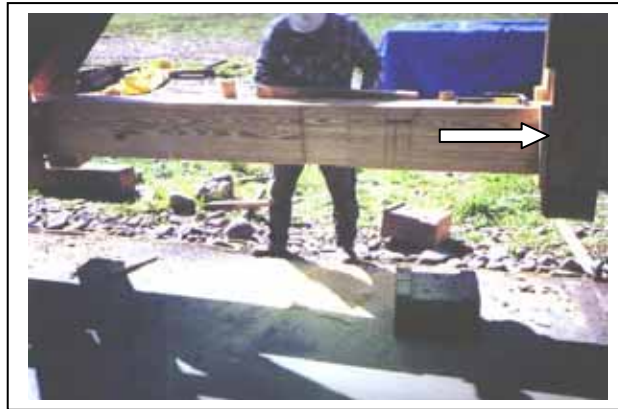
Figure 184. Wedges used in the connection between vertical post and chord—you have to look closely on the left side of the right post. In the writer's opinion, their value is principally to distribute the high side-grain bearing stresses in the post to a larger area.
