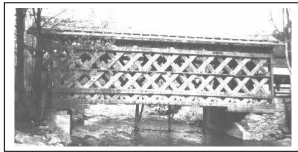
Figure 173. Side view of a typical covered bridge supported by Town lattice timber trusses. This is the Fuller Bridge, Montgomery, VT, during its recent reconstruction.
