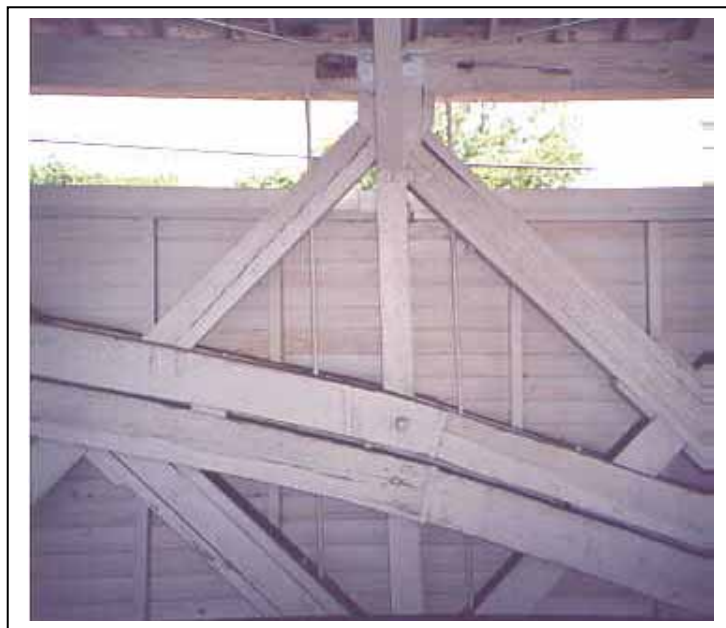
Figure 155. A single bolt connects these single-piece arch segments to the truss post—Wehr Bridge, Lehigh County, PA.
