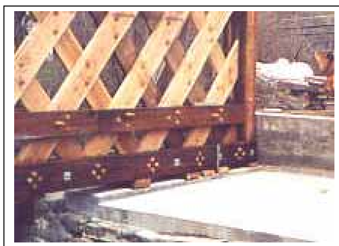
Figure 130. Bearing blocks beneath the bottom chord where tails have been removed—Paper Mill Bridge, Bennington, VT.
