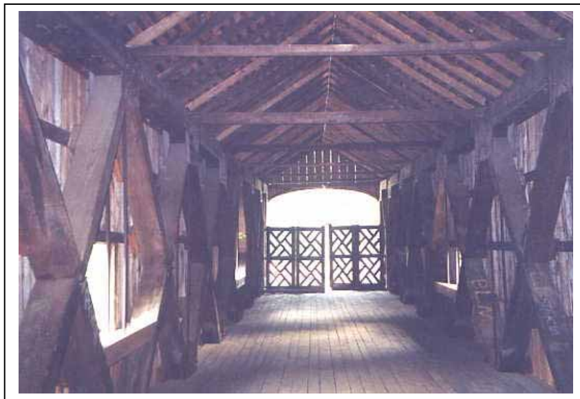
Figure 99. American Chestnut (allowable stresses are not in the NDS)—Comstock Bridge, East Hampton, CT.
