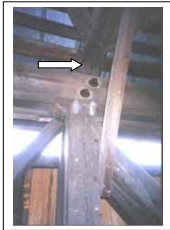
Figure 183. Diagonal to post connections at the top chord indicating significant overstress.
