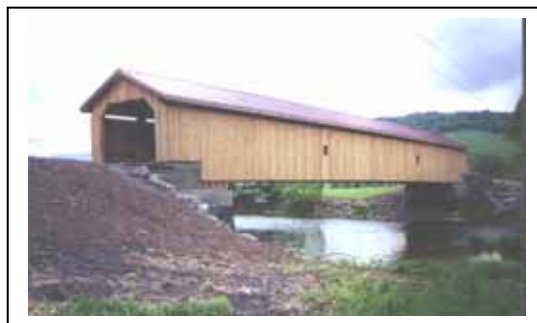
Figure 186. Near final exterior view. Guide rail not yet installed and final seeding and mulch also not yet in place.
