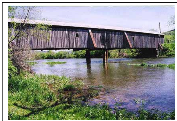
Figure 177. View of the Hamden Covered Bridge prior to work in 2000. Note the mid-span timber bent added in the 1970s to help support the sagging trusses. Also note the external top chord braces.
