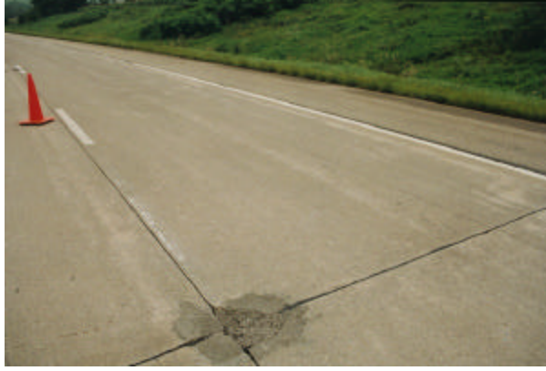
Figure 3.1.23 Corner break and repair at 27-4054.
