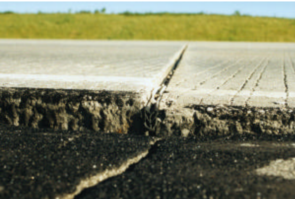
Figure 3.1.27 Transverse joint at 55-3008 (faulting of shoulder).
