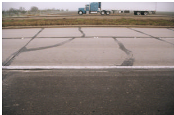
Figure 3.1.13 Corner break in truck lane at 06-CS3, Tracy Test Road (control section).
