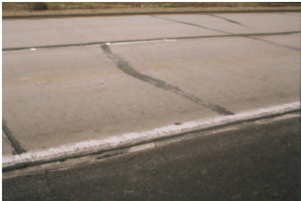
Figure 3.1.12 Crack only in truck lane at 06-CS3, Tracy Test Road (control section).
