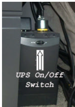
Figure 2.2.5.4. UPS on/off switch.
