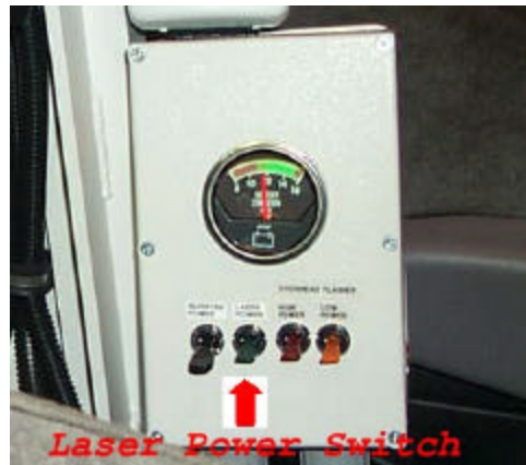
Figure 2.2.3.1. Laser on/off switch.
