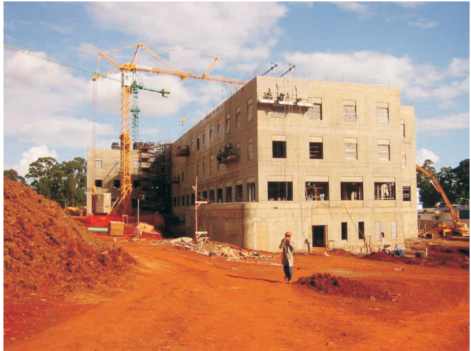
New U.S. Embassy in Nairobi, Kenya under construction after al Qaeda bombing.
