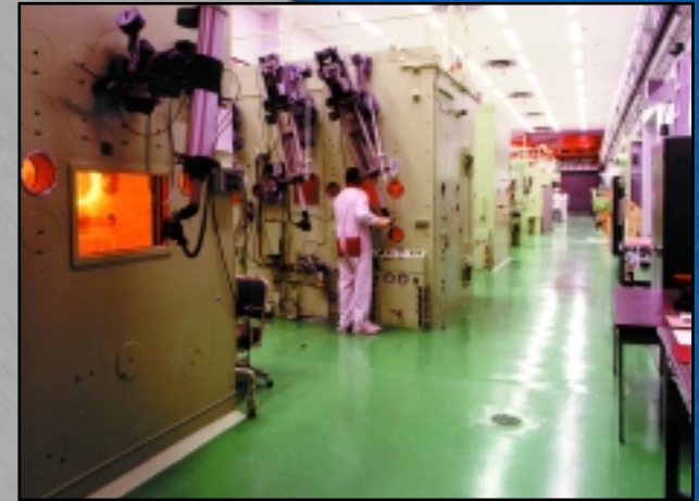
Hot cells line a corridor in the 327 Building. Three of the facility’s eight hot cells are now clean.
