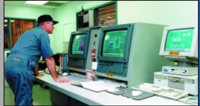
From inside the modern control room, an operator monitors treatment of wastewater at the 310 Treated Effluent Disposal Facility.
