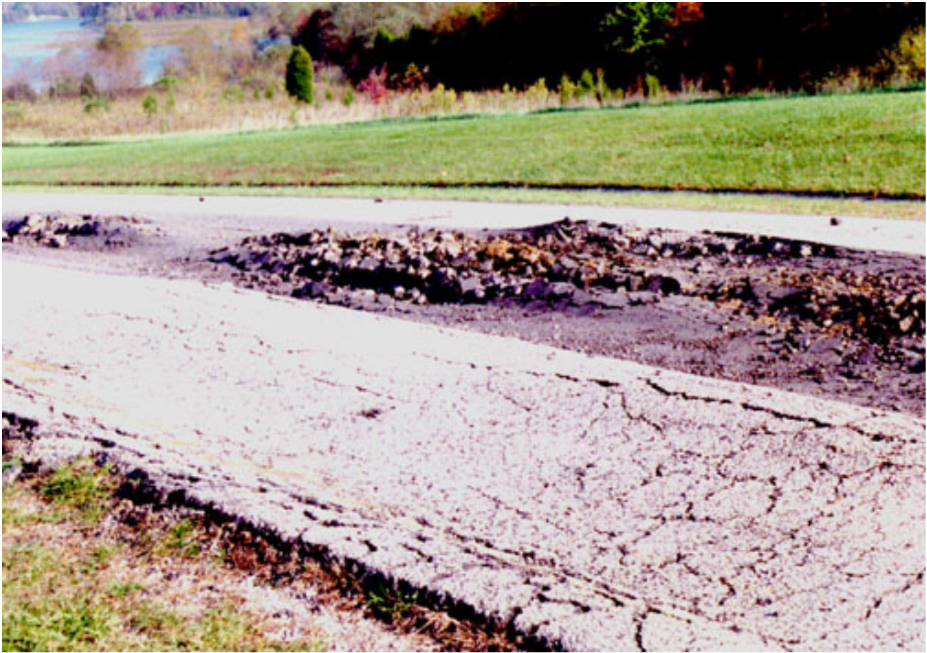
Figure 10.— Damage from frost heave has occurred to this road constructed in an area of Jennings soils. These soils have a high potential for frost action.
