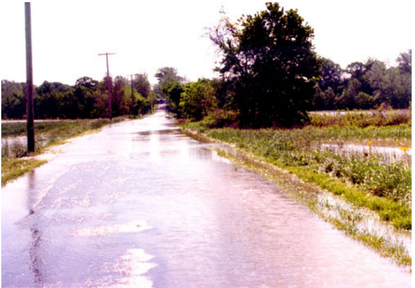
Figure 9.—Floodwaters cover this road that was built on Steff and Stendal soils. Building roads is a design concern for these soils and other flood plain soils that are subject to flooding.
