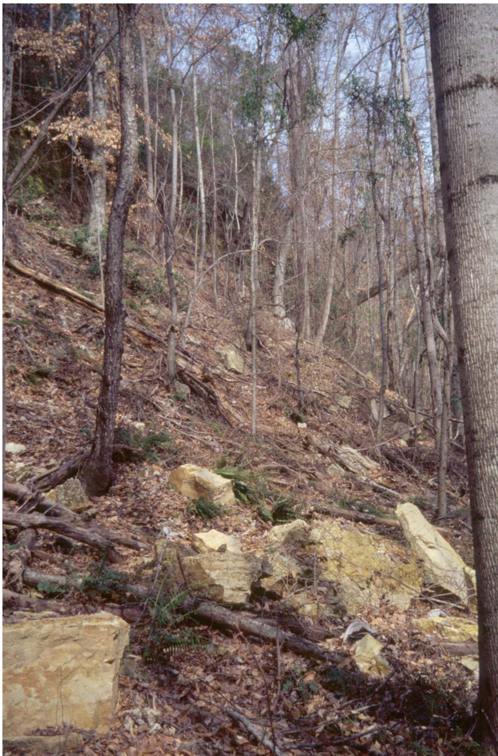
Figure 5.—An area of Arundel-Cantuche complex, 35 to 60 percent slopes, supporting a mixed stand of pine and hardwood. The curved and twisted tree trunks are a result of downslope movement and the compensating tree growth.
