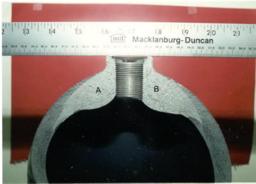
Figure 19: A macro view of the fracture surface. Side A was used for fractography and side B for metallography.
