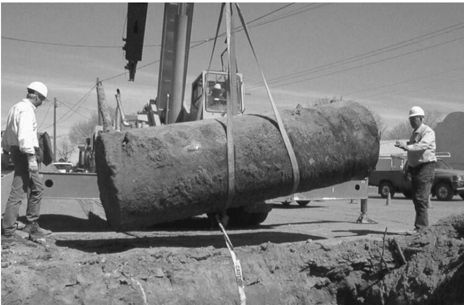
Removal of leaking underground storage tanks is one way to prevent groundwater contamination.
