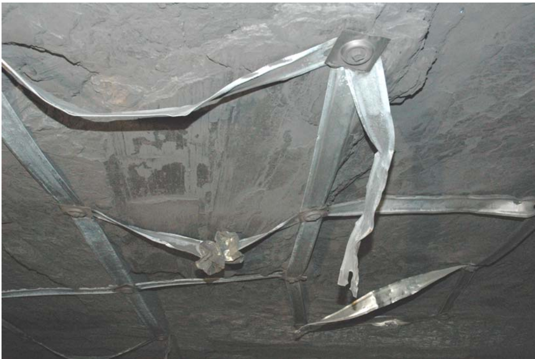
Photograph 12 - Damaged roof straps near A Left No. 3 Seal
