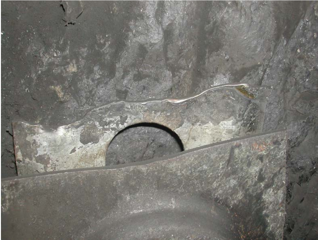
Photograph 7 - Outby segment of roof strap at A Left No. 3 Seal
