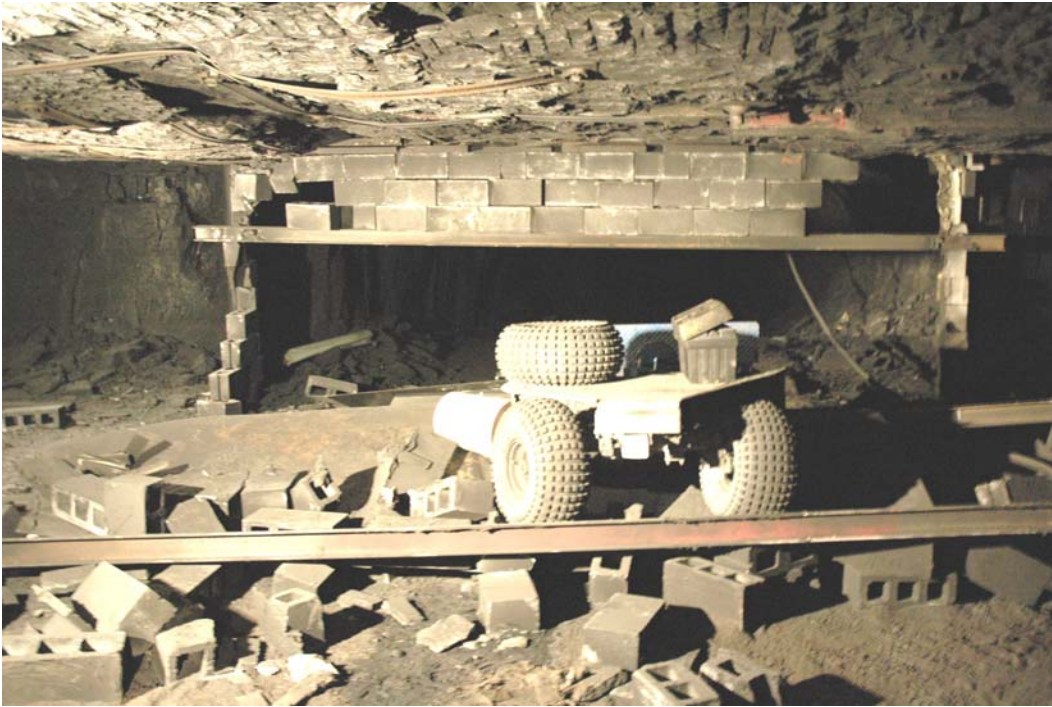
Photograph 1 - No.1 personnel carrier on damaged overcast
