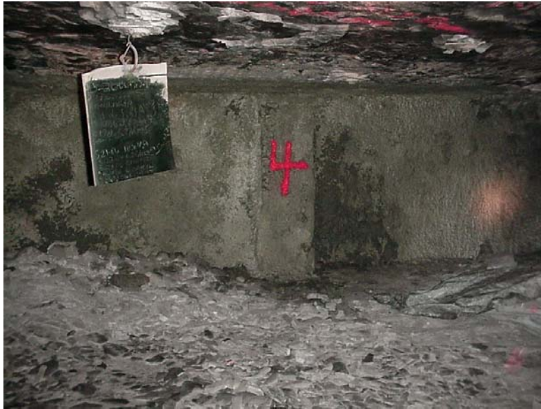
Figure 9 - No. 4 Intake Seal
