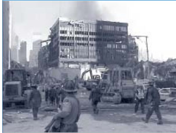
Photograph of the collapsed 6 World Trade Center building that TIGTA had occupied in New York City before the terrorist attack on September 11, 2001.
