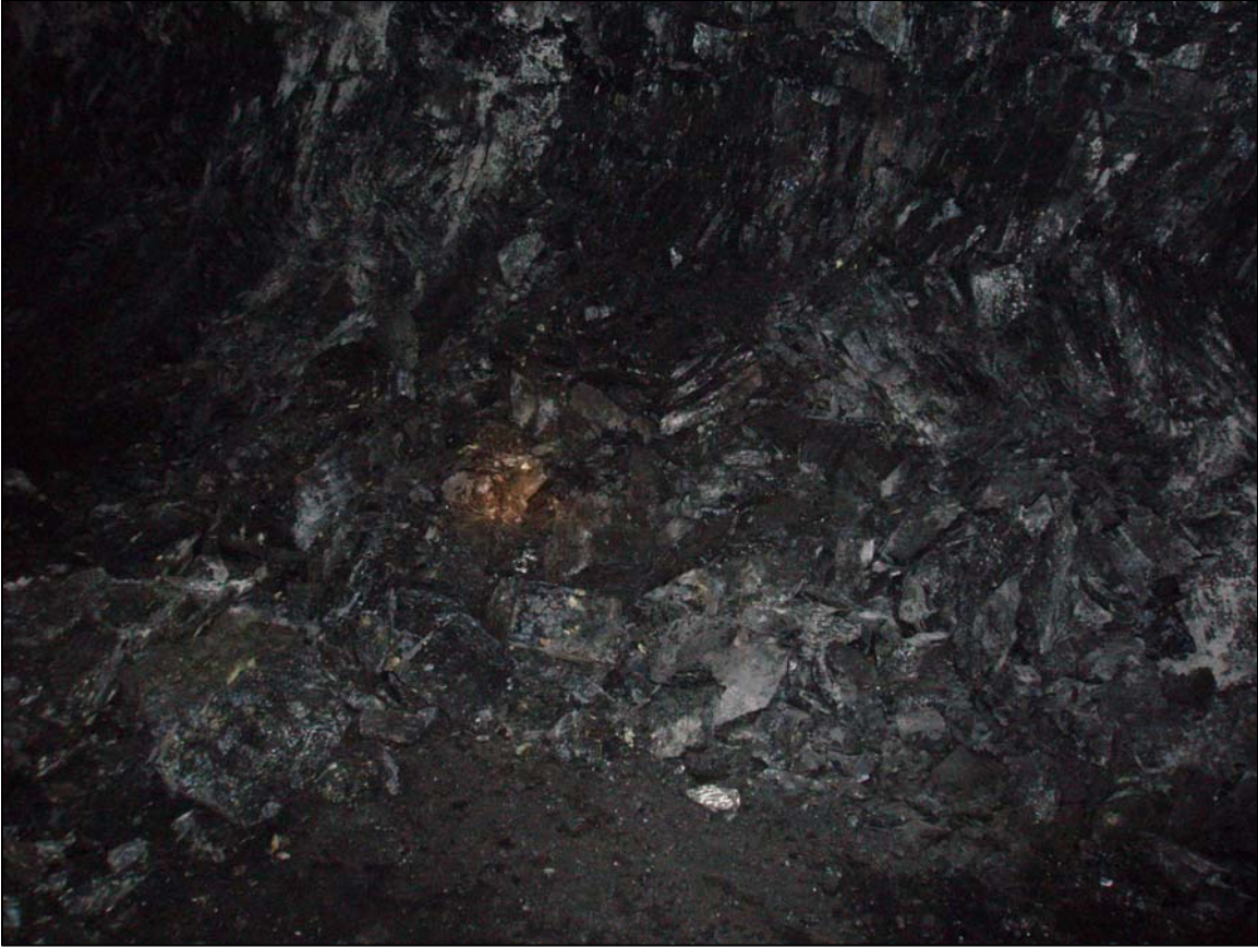
Photo 1. Rib Sloughing Near Crosscut 123 in the Entry North to the South Remnant Barrier Pillar
