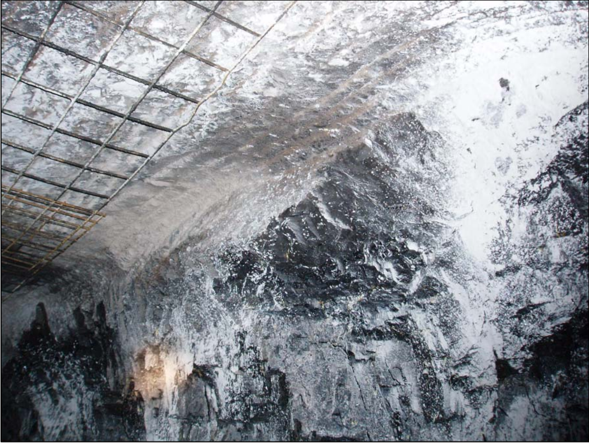
Photo 2. Minor Rib Sloughing at Crosscut 122 in the Second Entry from North Remnant Pillar
