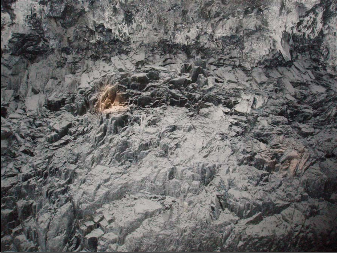
Photo 3. North Remnant Barrier Pillar Rib Condition Between Crosscuts 120 and 119
