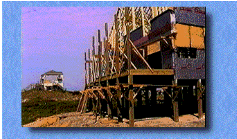
Photo 6. This house is being built on pilings to reduce potential damage from flooding and high waves.
