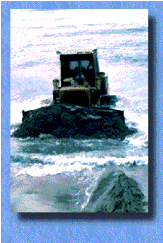
Photo 7. A bulldozer pushes sand onto the beach to rebuild the dune that helps protect the property behind it.
