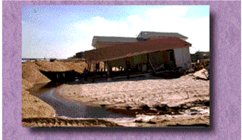
Photo 12. The storm surge from Hurricane Fran collapsed many buildings built prior to 1985.
